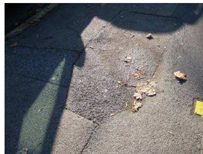
Figure E.5: Irregular footway surface
