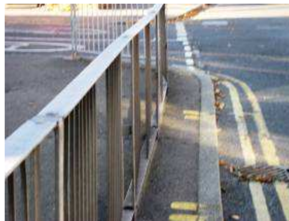
Figure E.6: Double Yellow lines and pedestrian railings on South side of the junction
