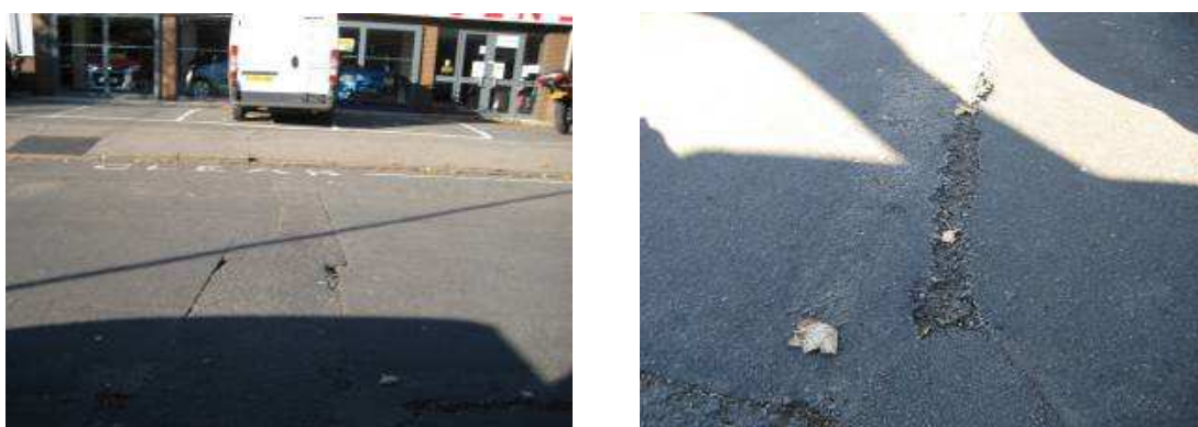
Figure E.9(a) and E.9(b): Carriageway surface on Holme Lacey Road
