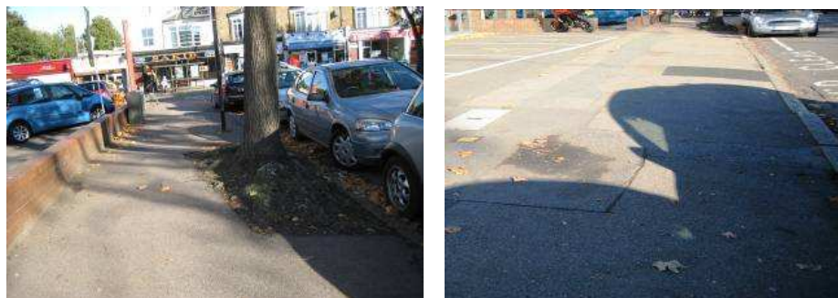
Figure E.8(a) and E.8(b): Footway surface Holme Lacey Road, North side
