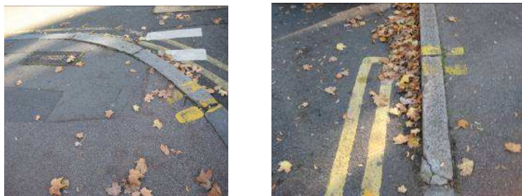
Figures E.1 (a) and E.1 (b): Double yellow lines and pips at the corner of the junction
